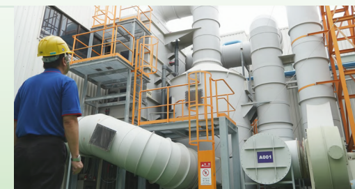
Wet Scrubber Processing Equipment
