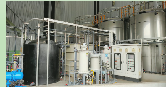
Waste Acid Recovery System
