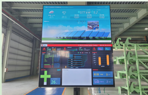
Douliou Mill II Power Generation Monitor
