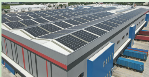
Mill Rooftop Solar Power Panel
